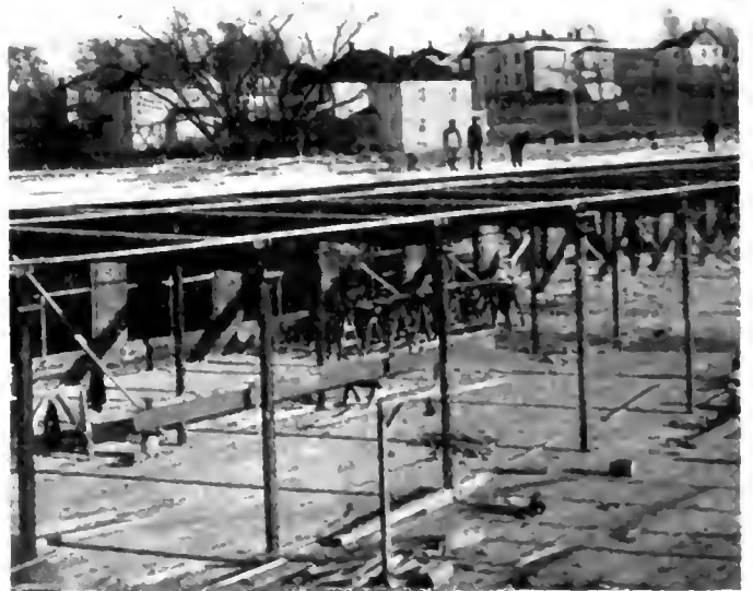
Fig. 3—Steel work proceeding for the third floor. Cast iron columns and I-beams are used with timber floors.
